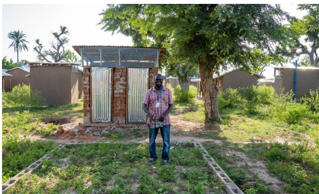
Mustapha Shuaibu, IOM Water and Sanitation Hygiene Operation Facilitator, stands in a space designated for a family's home in Malkohi. Behind him is the home's latrine, under construction.
